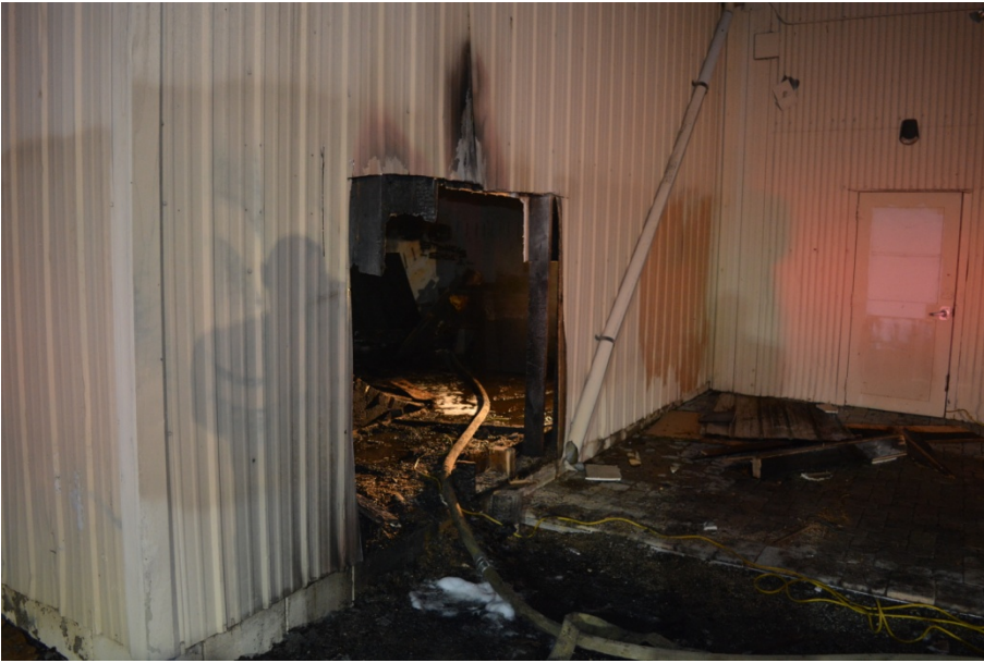
265 Keystone Fire Damage Photos
